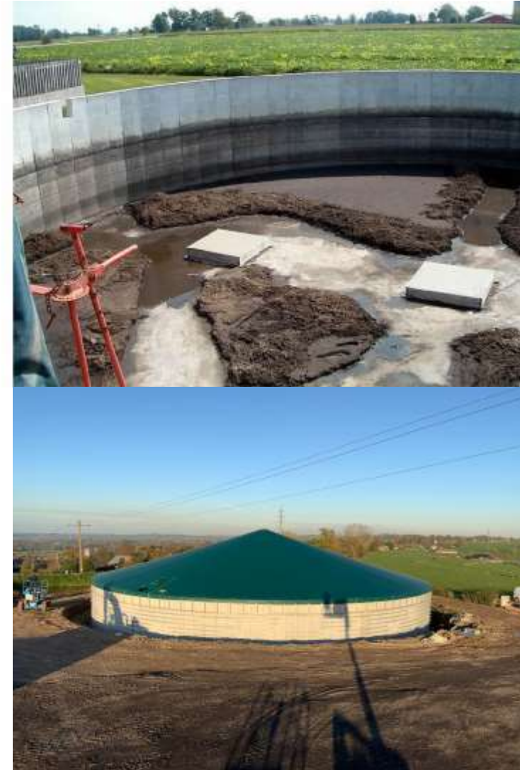
Manure storage tank
