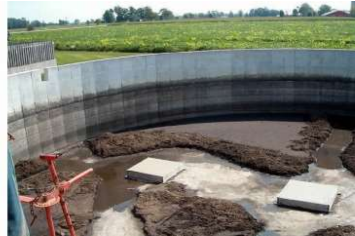
Manure storage tank
