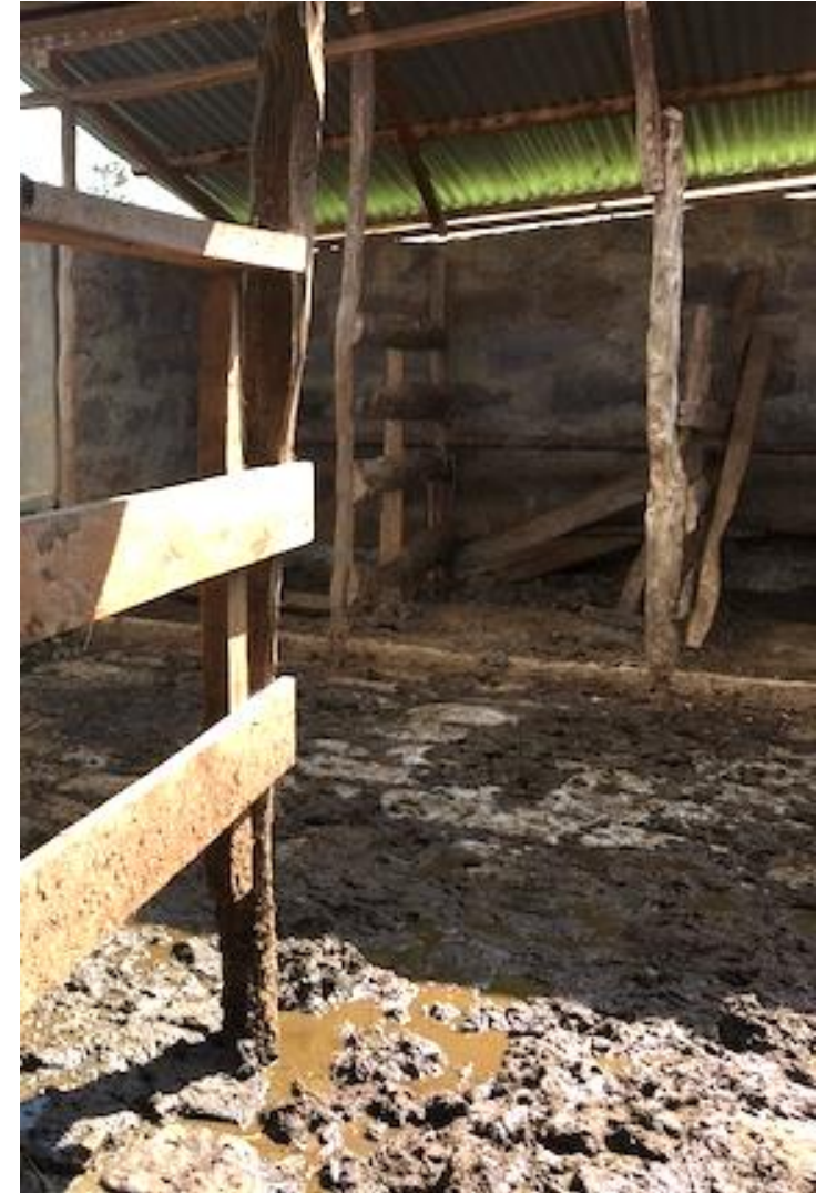
Too rough floor with poor drainage of slurry
