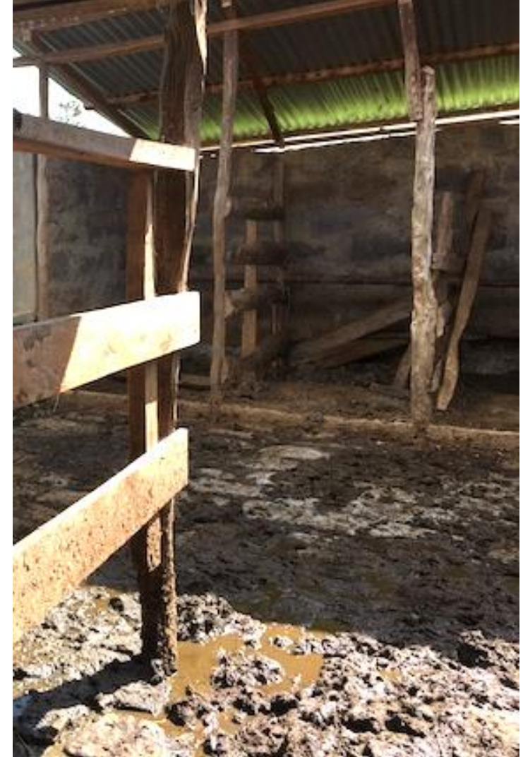
Too rough floor with poor drainage of slurry
