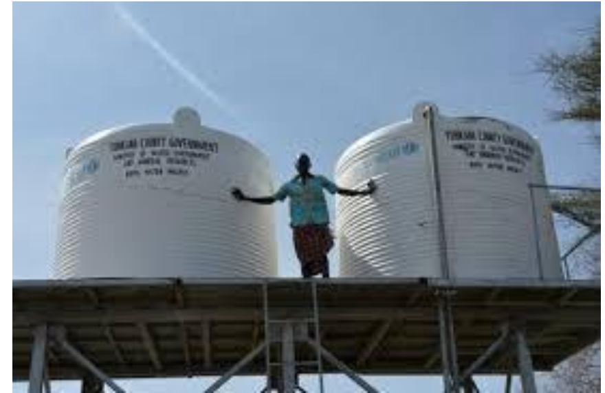
Elevated plastic tanks
