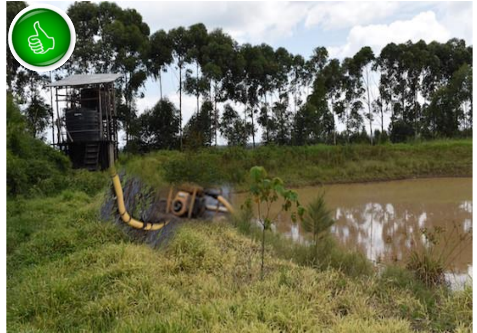
Water pumped to overhead tank
